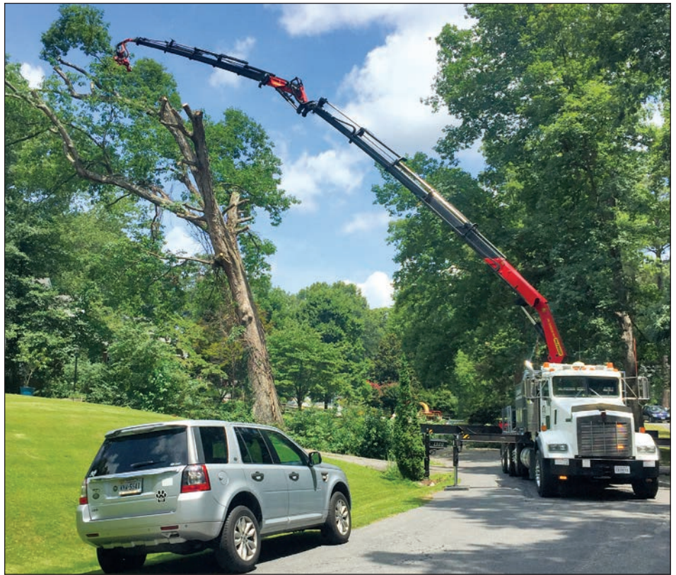
The time it takes to process big stick-crane picks with minimal manpower and equipment isn't any more efficient than using a grapple saw to strategically dismantle the tree into manageable pieces at a steady rate.
